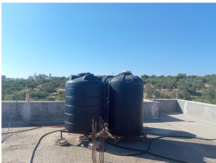
Figure 4 | Cold water tanks. Source: Photo by Saara.
